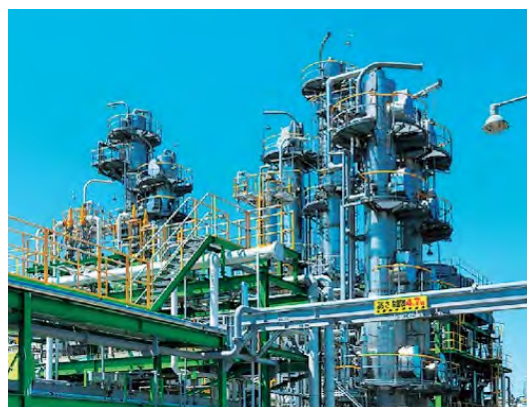
Koshijihara Plant, Nagaoka Field
