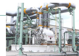
Demonstration facility of Centrifugal hydrogen compressor
