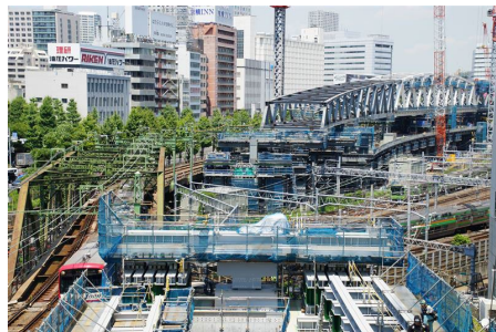
Replacement of the Yatsuyama Bridge between Shinagawa and Kita-Shinagawa on the Keikyu Main Line, spanning 10 JR lines
