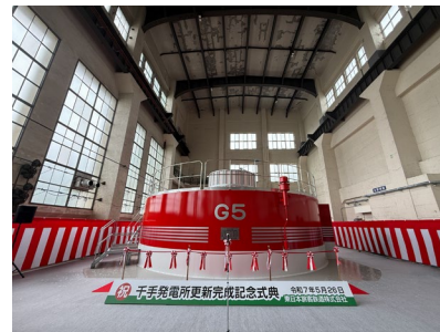
Equipment renewal work at JR East Shinano-gawa Power Station (Senju Power Station)
