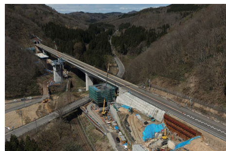
Example of construction at an intersection between a railway and a road
