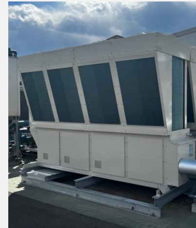
Air-cooled heat pump chiller
