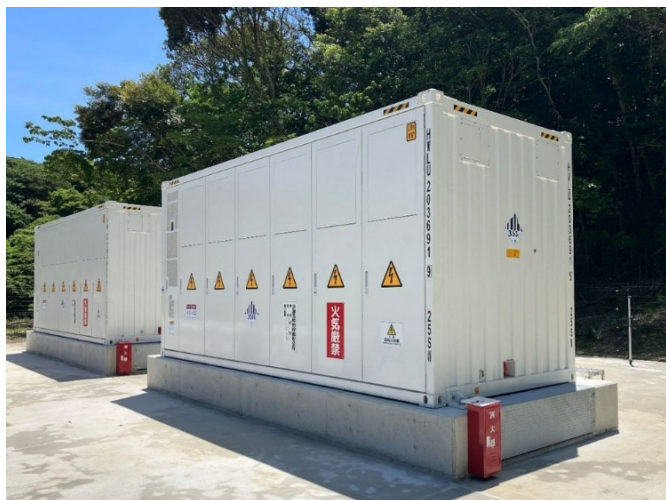
Ichigo Onjuku Iwawada ECO Battery Storage Plant
