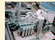
Large-scale hydrogen production facility
