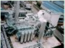
Large-scale hydrogen production facility (Our EPC)
