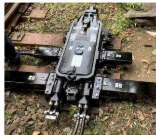
Replacement with water-resistant electric point machines
