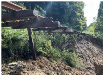
Washout of trackbed
